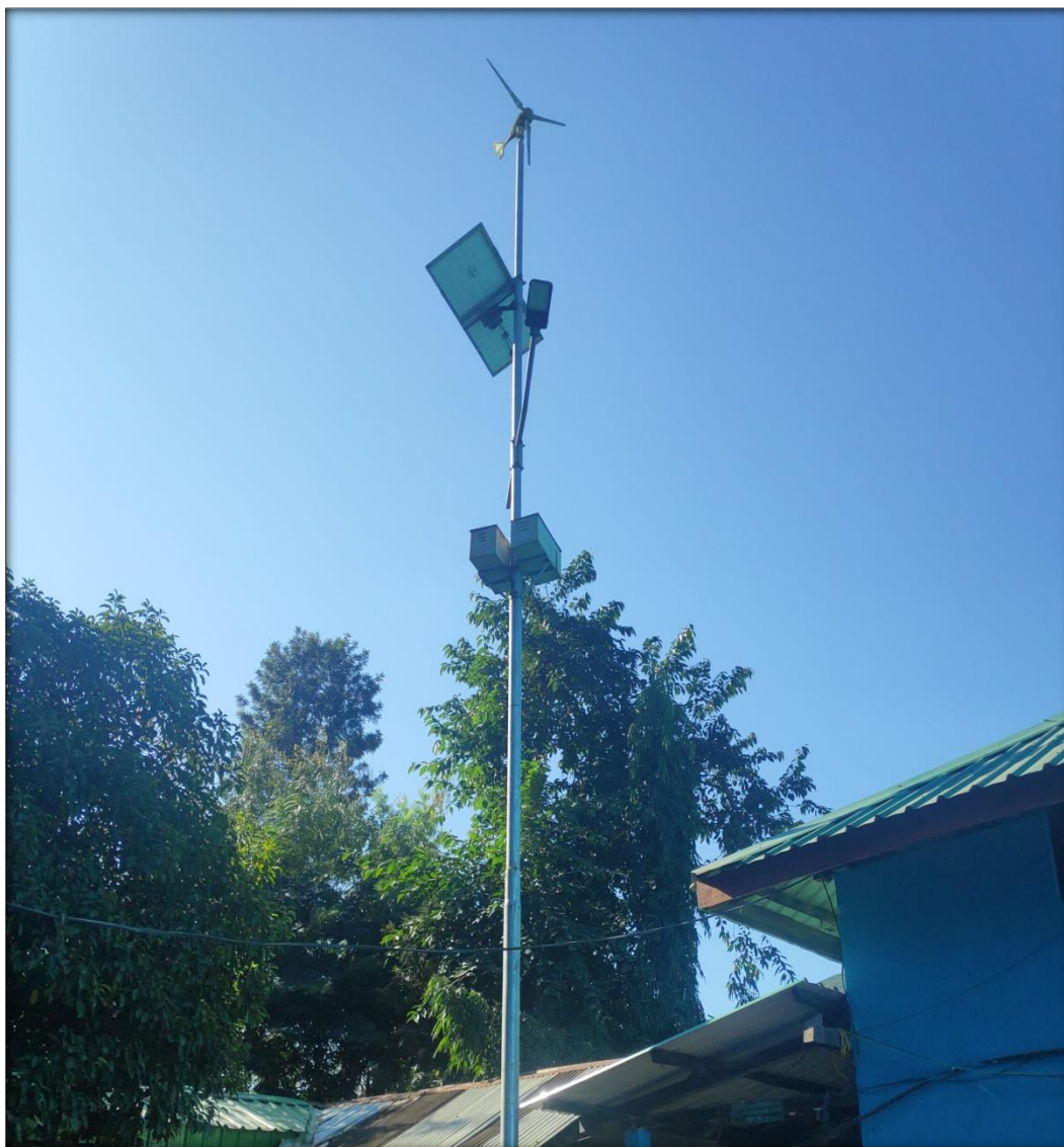
Fig 14: A LED Wind Solar Hybrid Street Light
